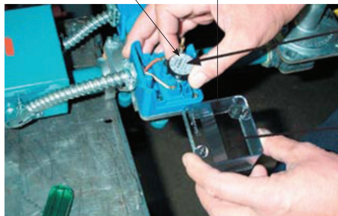
Gas pressure switch adjustment – Type A
