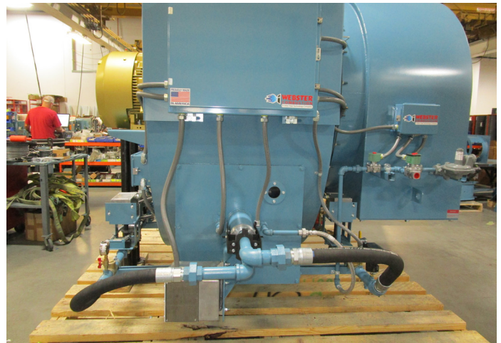
Rear-mounted junction box exterior
