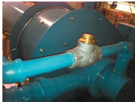
Figure B-14.1 Center Gas Balancing Valve
