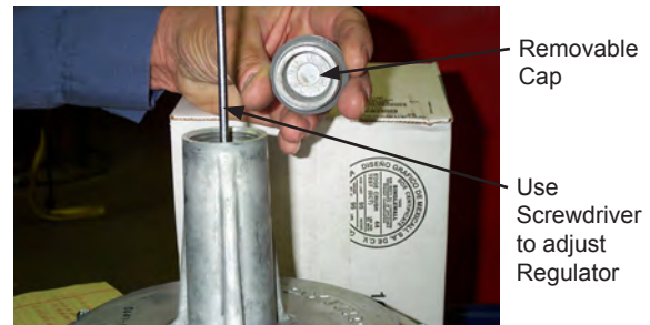
Figure E – 7 Main Gas Pressure Regulator Adjustment
