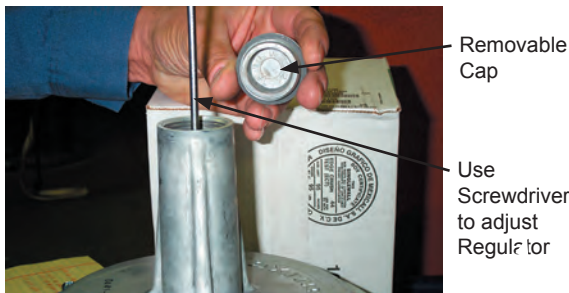
Figure E-9 Main Gas Pressure Regulator Adjustment
